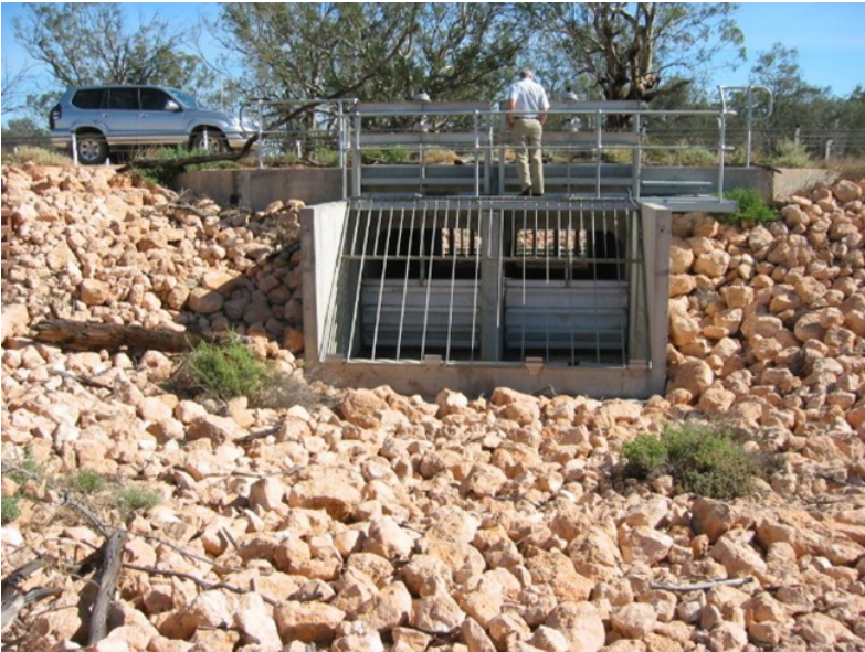
Photo 1: An example of an existing regulator and spillway at Lake Wallawalla West (Credit: Mallee CMA)
